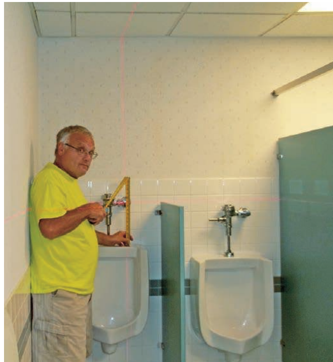
▶ Mark Kidd, owner of the Kidd Plumbing in Allentown, Pennsylvania, uses a Spectra Precision 5.2XL laser level during the installation of plumbing fixtures. (Photo courtesy of Kidd Plumbing)
