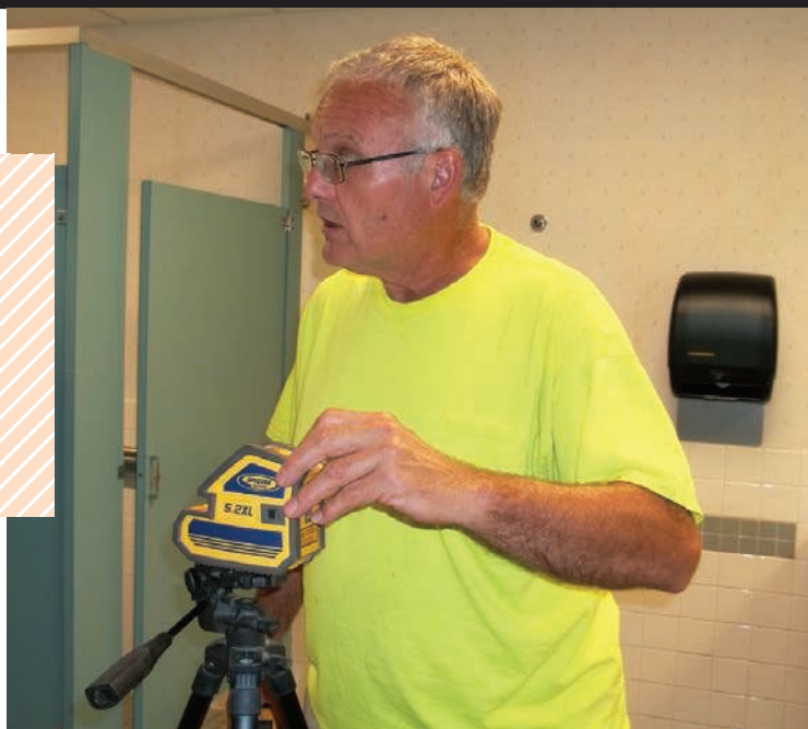
▲ Mark Kidd, owner of the Kidd Plumbing in Allentown, Pennsylvania, uses a Spectra Precision 5.2XL laser level during the installation of plumbing fixtures.
