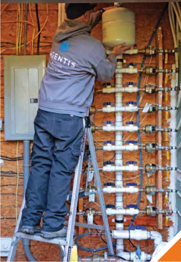
▲ Plumber Dan Thomas removes a thermal expansion tank as the team works on replacing them with newer tanks.
